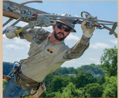
MEDIUM & HIGH VOLTAGE
